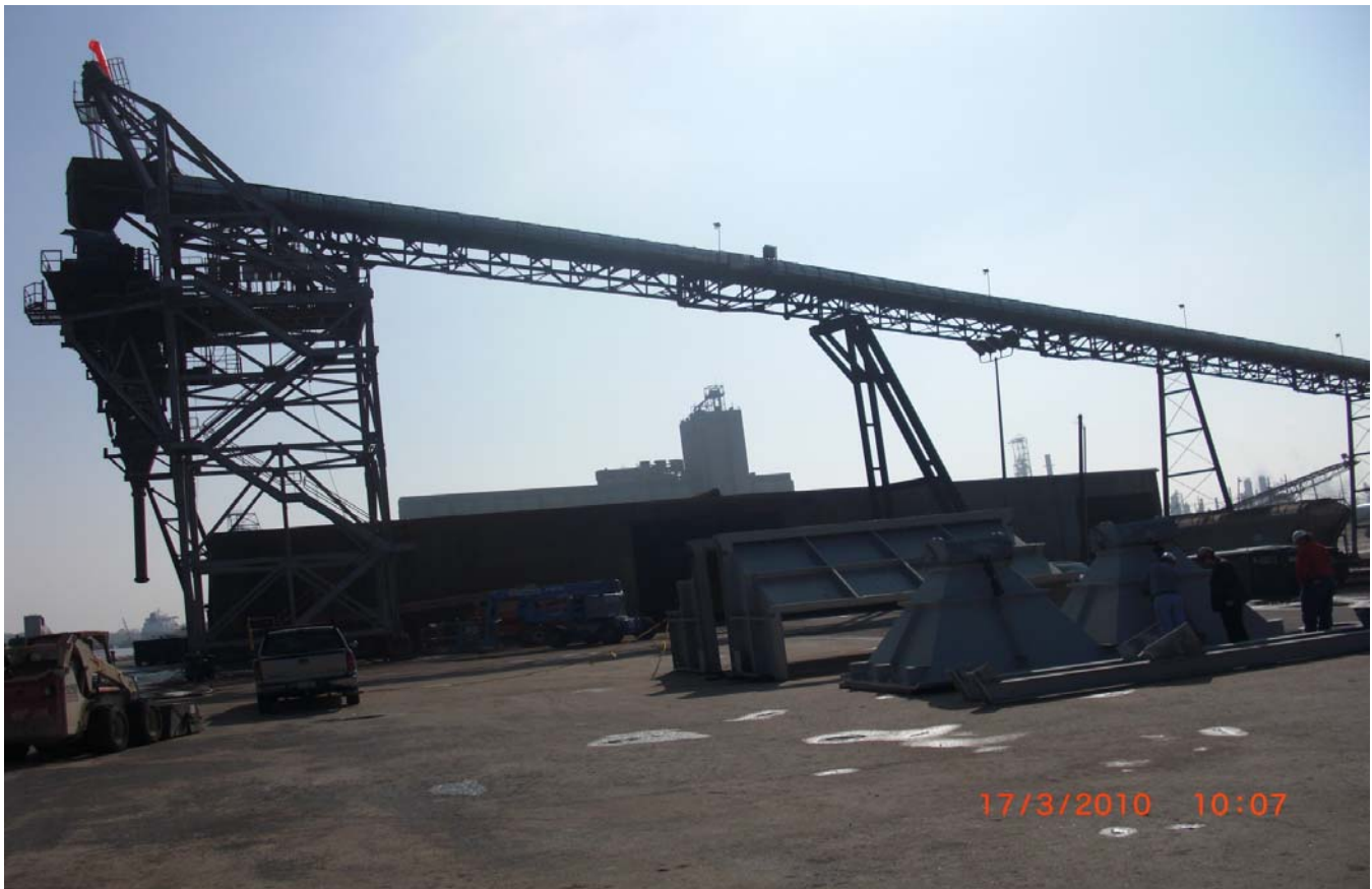
Ship Unloader – General View
