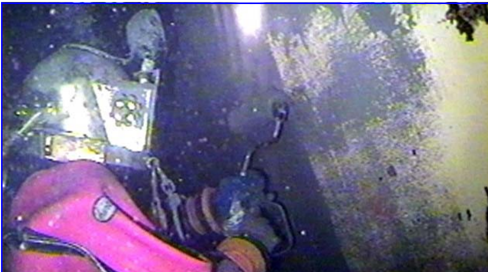
This guy is underwater! A UCC diver rolls on a coat of special epoxy to a wall of the Unit 1 Spent Fuel Pool. The epoxy, which will prevent the release of airborne contamination once the pool is drained, is applied by divers while they are submerged underwater.
